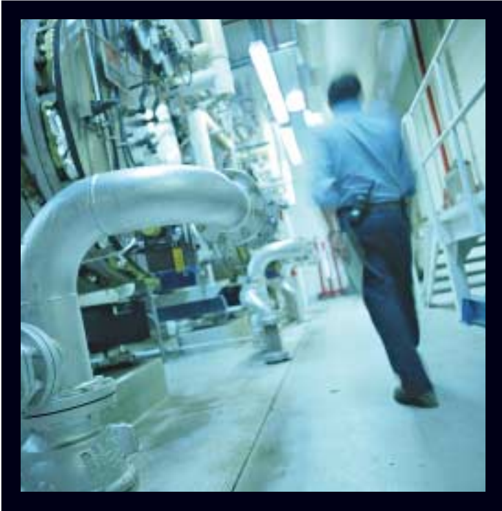
Twice a day, engineer Les Wittmeier or one of his colleagues inspects the biowaste system at the Winnipeg complex. It provides secondary treatment for about 13,000 litres of effluent a day. Primary treatment occurs in the lab. When sterile, liquids are discharged into the municipal sewer.
